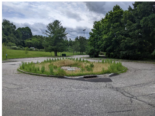
FocalPoint Bio-infiltration: SE-EB-715
