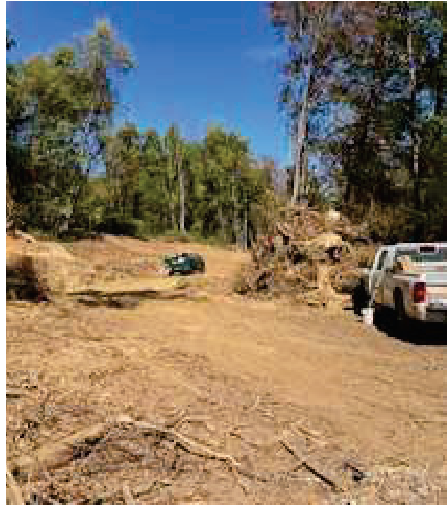
Stabilization Installation: Kent-MB-1000
